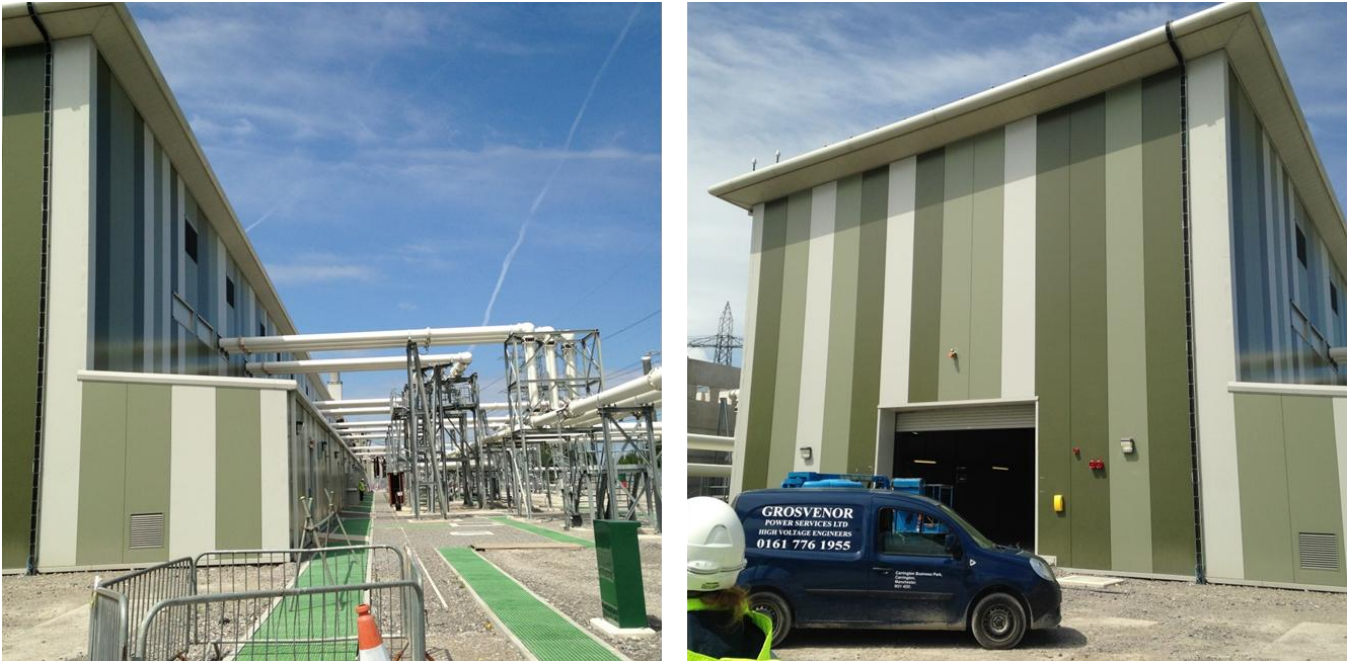
Image 3.6 and 3.7 National Grid Deeside Centre for Innovation 400 kV Substation (Source: National Grid)
