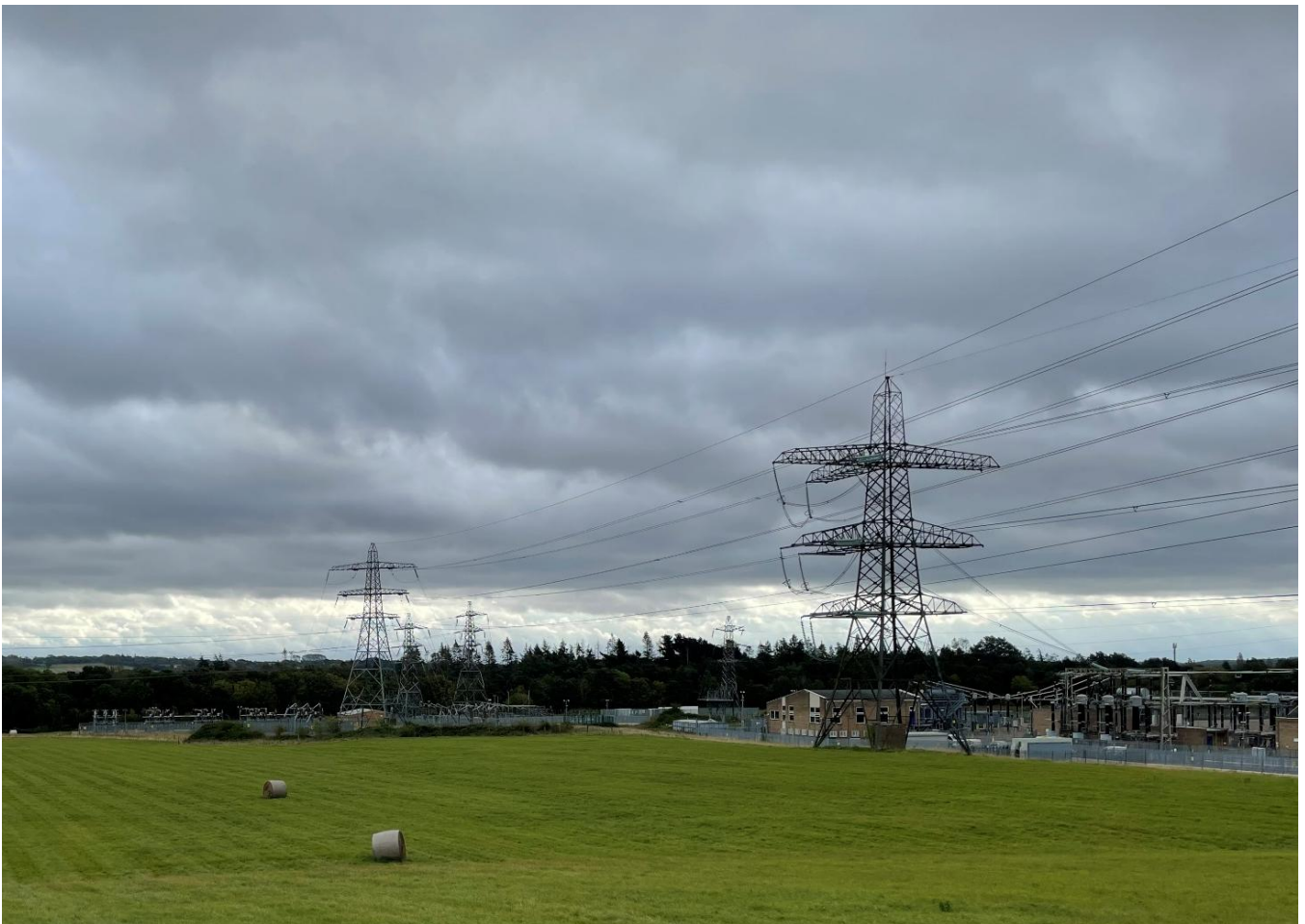
Image 3.1 Existing Norwich Main Substation 400 kV (Source: Norwich Main Site Visit)
